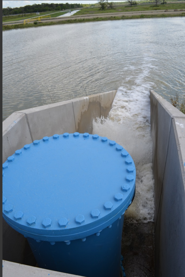
SB3, 4, & 5 INFLOW STRUCTURE
