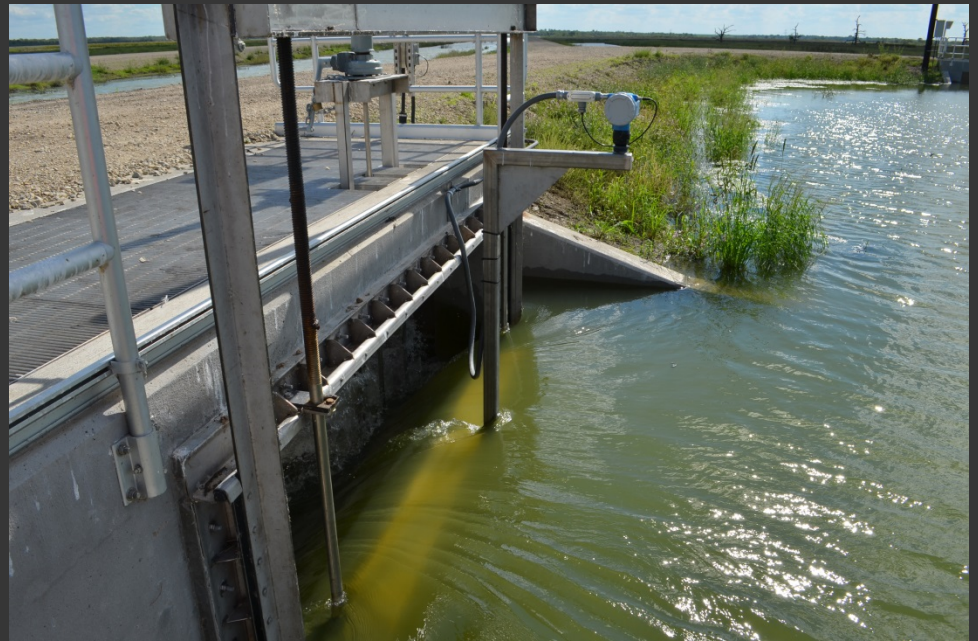
COLLECTION POOL OUTFLOW STRUCTURE
