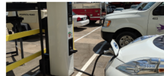
City of Lewisville's DCFC Charging Station on Their Fleet Lot.
