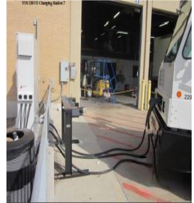
Terminal Tractor, Connected to Charging Unit
