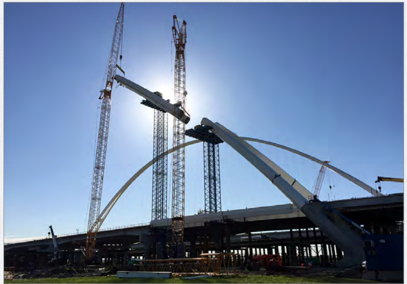
Pictured above is the construction of the westbound arch of the Margaret McDermott Bridge on the Horseshoe Project.
