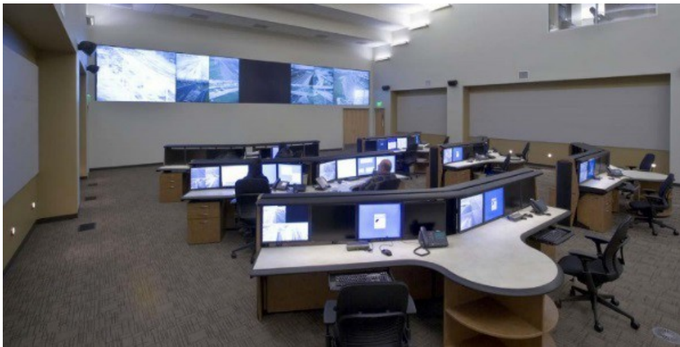
TxDOT Dallas District TMC
