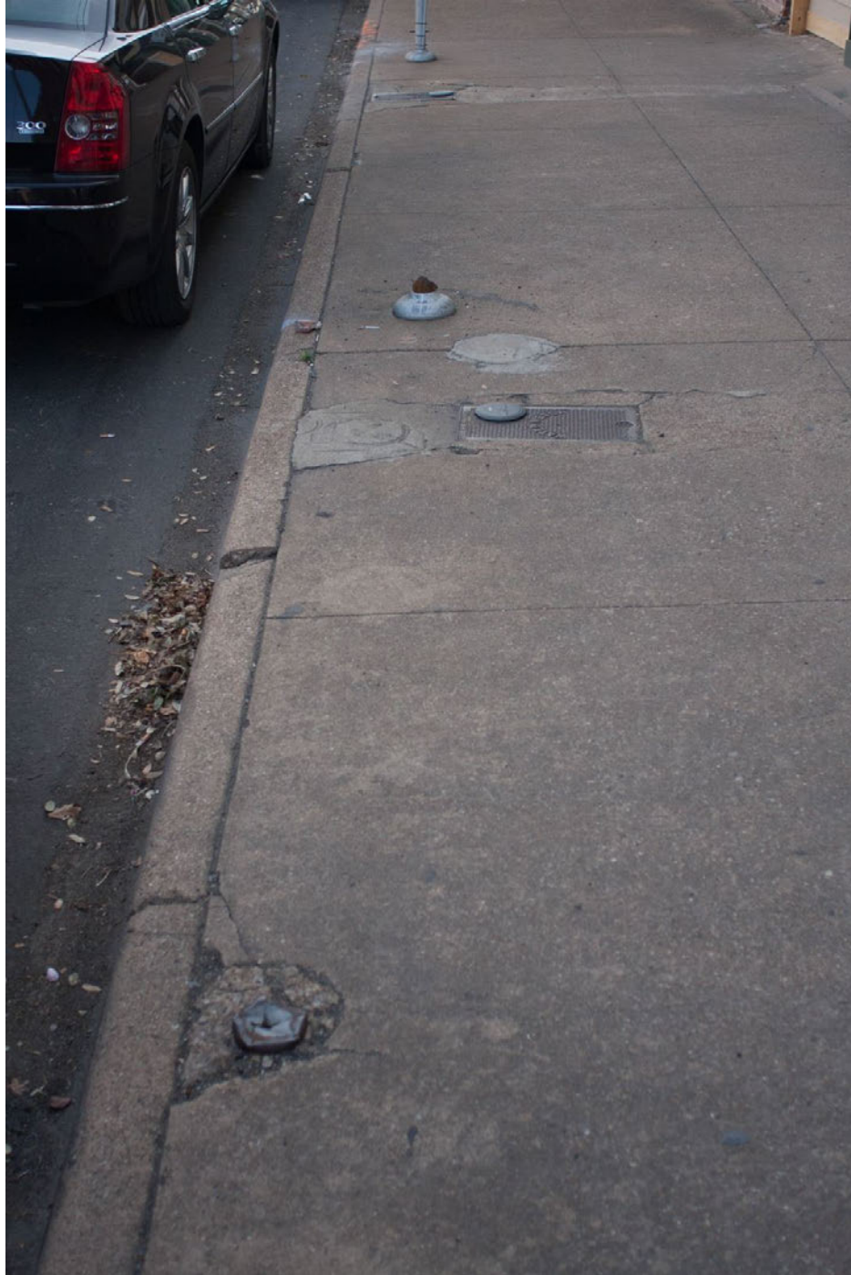
Throughout the area, utility meters, grates, stumps where parking meters formerly stood, and other surface obstacles present potential accessibility and aesthetic issues. Location: non-specific.
