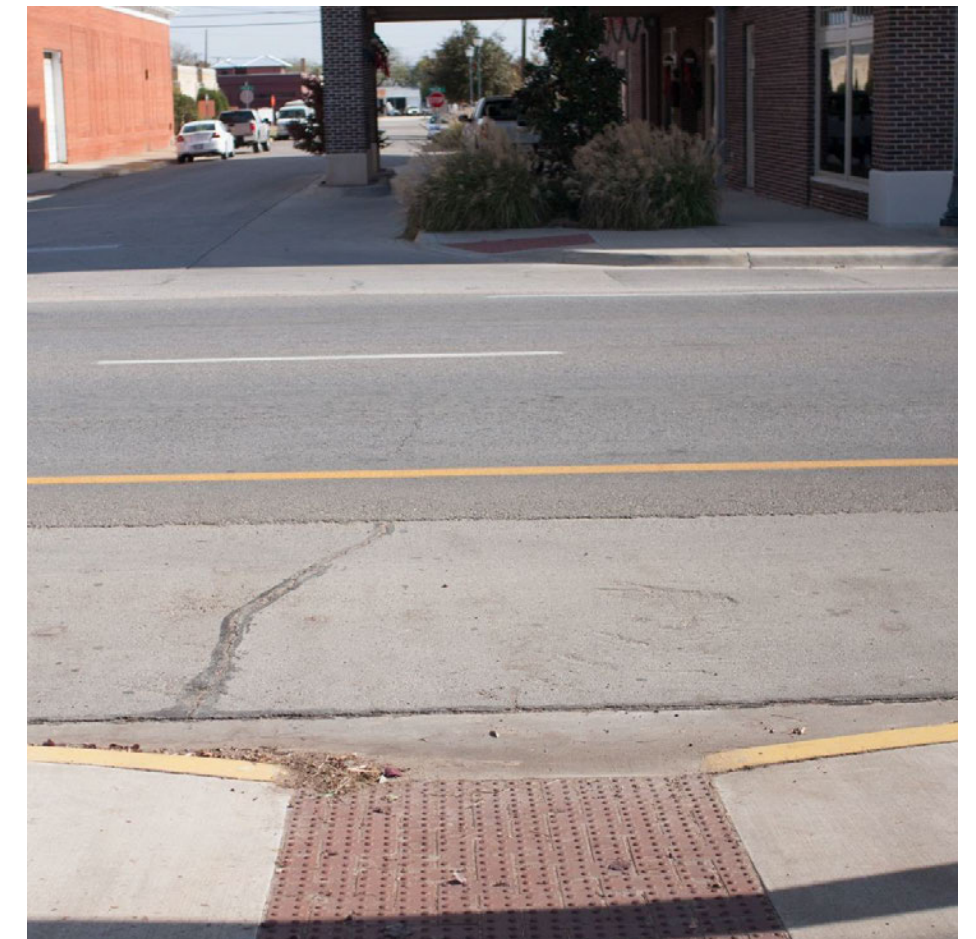
New sidewalks were built around the Wright Place building. These represent the most-accessible sidewalks in the best condition. However, there are instances where marked crosswalks and no-parking zones are missing, rendering curb ramps ineffective. Location: Caddo Street at James Street
