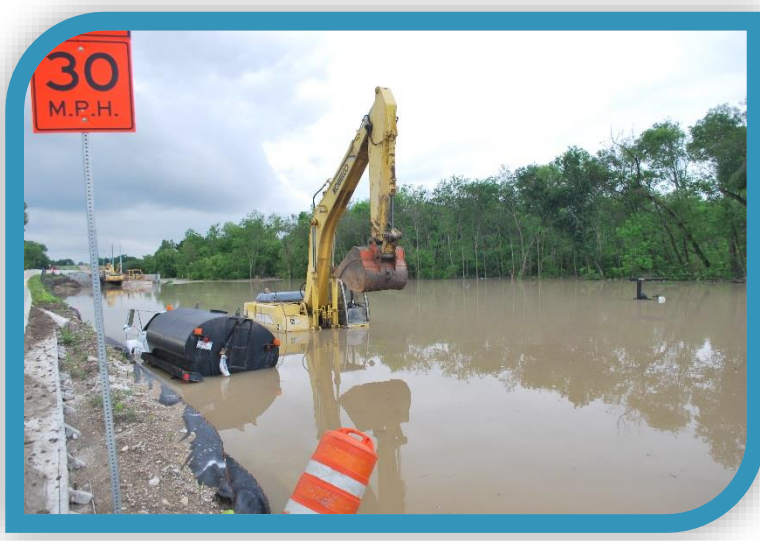
J. Rowlett Creek at Miller Road, Rowlett, Texas Credit: Dennis Abraham, NCTCOG Flood Photo Library
