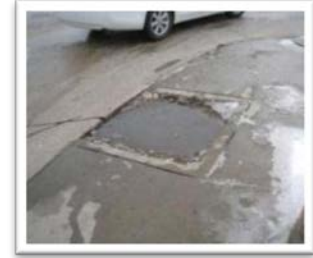
Figure 29: Hole at SW Corner of Park Lane and Shady Brook
