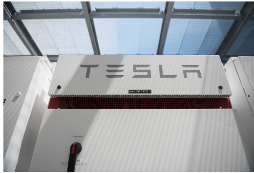
Battery Energy Storage
