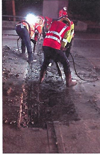
Dallas District maintenance crew conduct night repairs to a bridge joint at US 175 and I-20.
