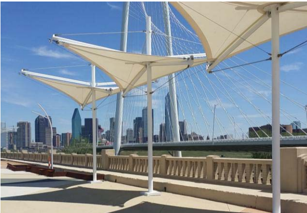
The Continental Bridge, a former vehicular bridge, is nearing completion as a dedicated pedestrian and bicycle facility and will provide access to Downtown from the Trail.
