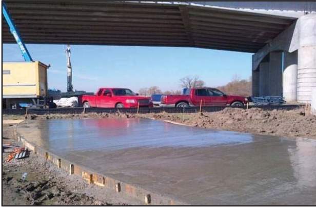
Section of the Trinity Skyline Veloweb Trail under construction south of the Sylvan Ave. bridge. The proposed TIGER project will extend the trail northward.
