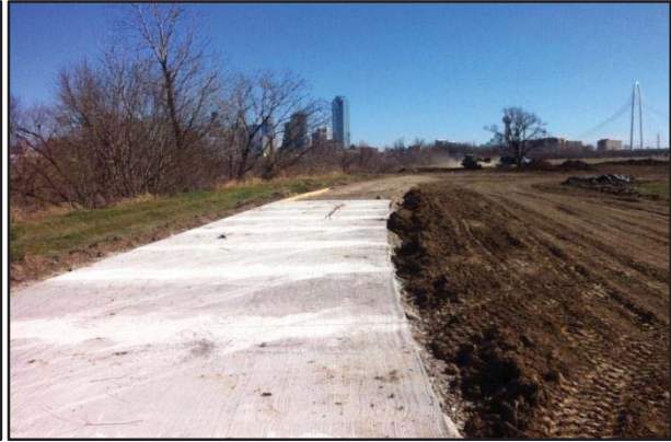
Section of the Trinity Skyline Veloweb Trail under construction (view from near the Sylvan Ave. bridge south towards Downtown Dallas).
