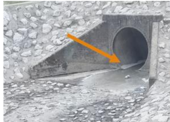
Staining in outfall from concrete washout
