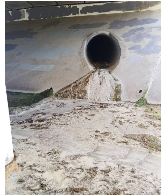
White deposits from gypsum plaster discharge
