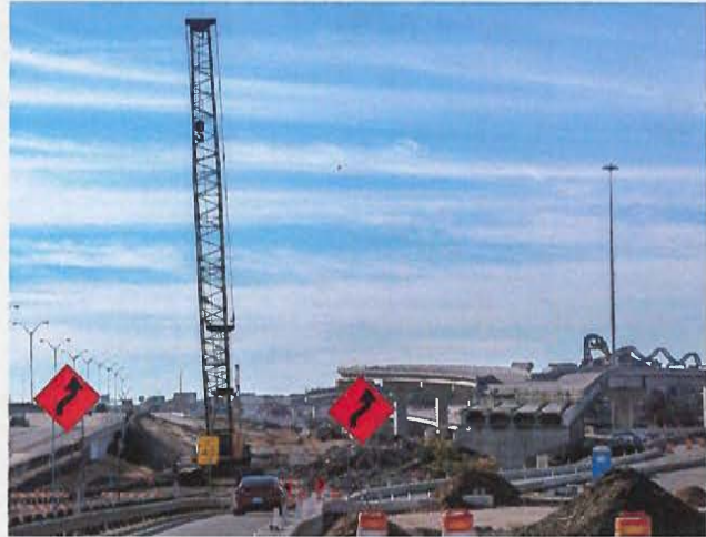
Construction on the I-30/SH 360 Interchange Project in Arlington. The $233 million project will increase safety, connectivity and mobility for motorists.
