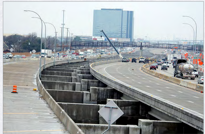
Looking westbound at the construction on the depressed TEXpress Lanes on LBJ Express looking west at the Rosser Road pedestrian bridge.
