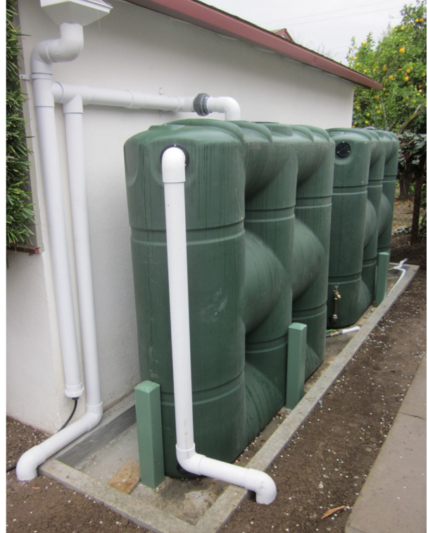
Rainwater Harvesting in Los Angeles, CA. (Source: Tetra Tech)
