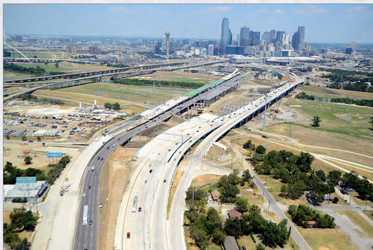
Pictured above is an aerial view of the Horseshoe construction progress on I-35E from south of Colorado Boulevard looking north toward downtown Dallas.
