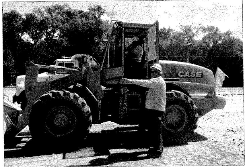
Jason Palmer and Kent Rivers of TxDOT's Denton Area Office work with the Texas Department of Parks and Wildlife to remove 1,110 tons of silt and dirt from parking lots and roads in the Greenbelt Corridor of Ray Roberts Lake State Park.
