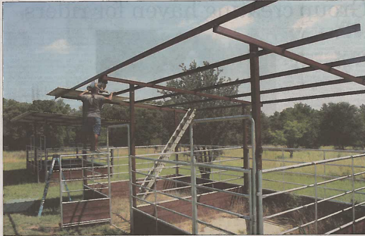
Damon Brown works on a horse shed with his daughter, Shanika Allen, at the Bluestem Grove area of Ray Roberts Lake State Park. The sheds are being built by members of the Lake Ray Roberts Equine Trail Association.
